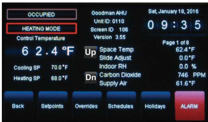
Figure 15: DDC Controller Status Screen 1
