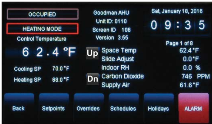
Figure 21: DDC Controller Status Screen
