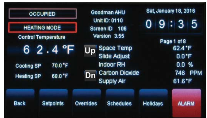
Figure 14: DDC Controller Status Screen 1
