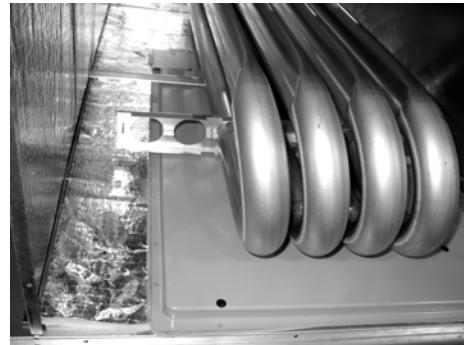
Figure 19: Discharge Panel In Place
